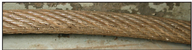
Outside of wire rope. It appears to be in good condition. See below.
